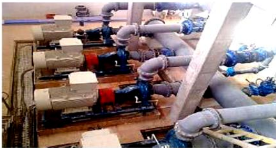
Fig. 2. Electropumps available at the station.
