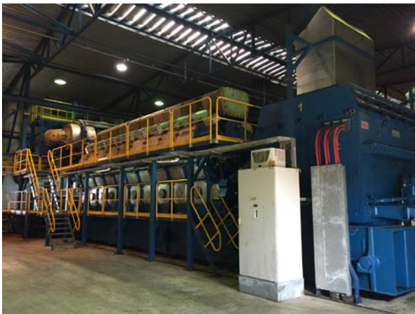
Figure 2. Diesel Generator n° 3.
